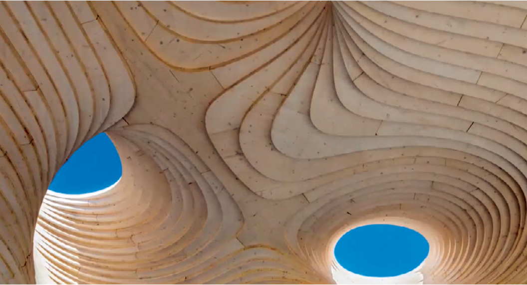
The CLT ceiling of Mill River Carousel Pavilion in Stamford, CT. Photo courtesy of Gray Organschi Architecture/Structure Fusion.
