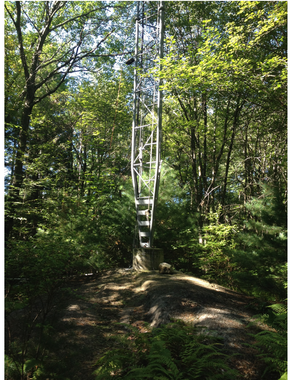
View of the base of the tower, with a deep concrete foundation to keep it in place.
