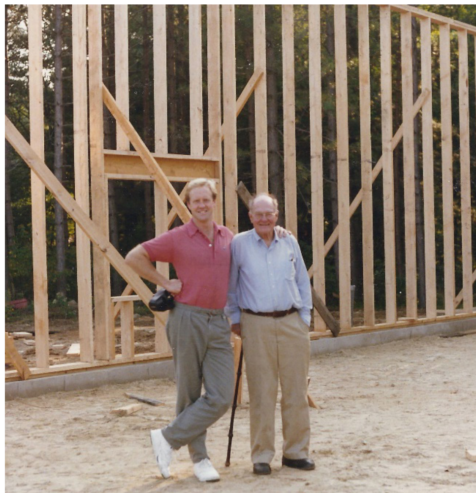
Starling and Ted Childs, standing by the frame of the new Forestry Office, circa 1990.
